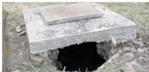
Example of an uncovered Abandoned well
